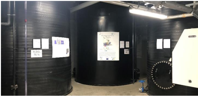
Chemical tanks and acidification
