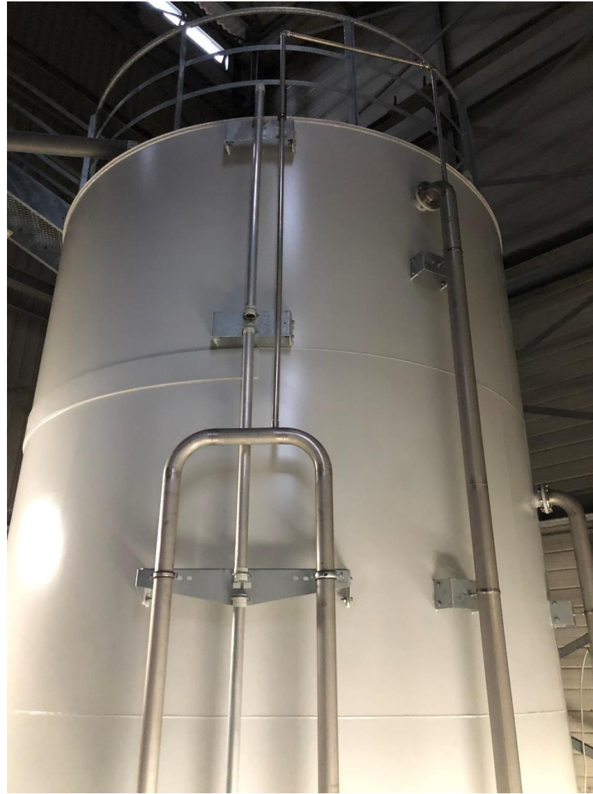
Reactor with discharge pipe system
